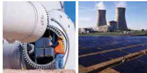
Operators assembling a turbine rotor at ground-level, before it is lifted on to the tower at the Cedar Creek Wind Farm in Weld County, Colorado, US.
