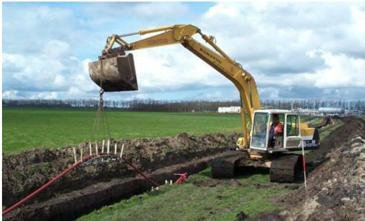
Figure 10: Typical crane with a quadrant
