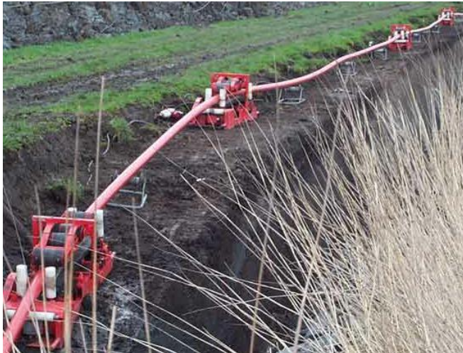
Figure 8: Typical cable tensioners
