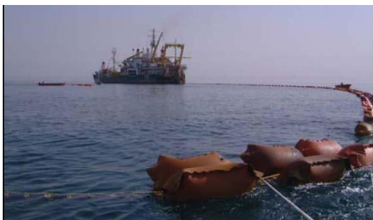
Figure 15: Cable with cable floats
