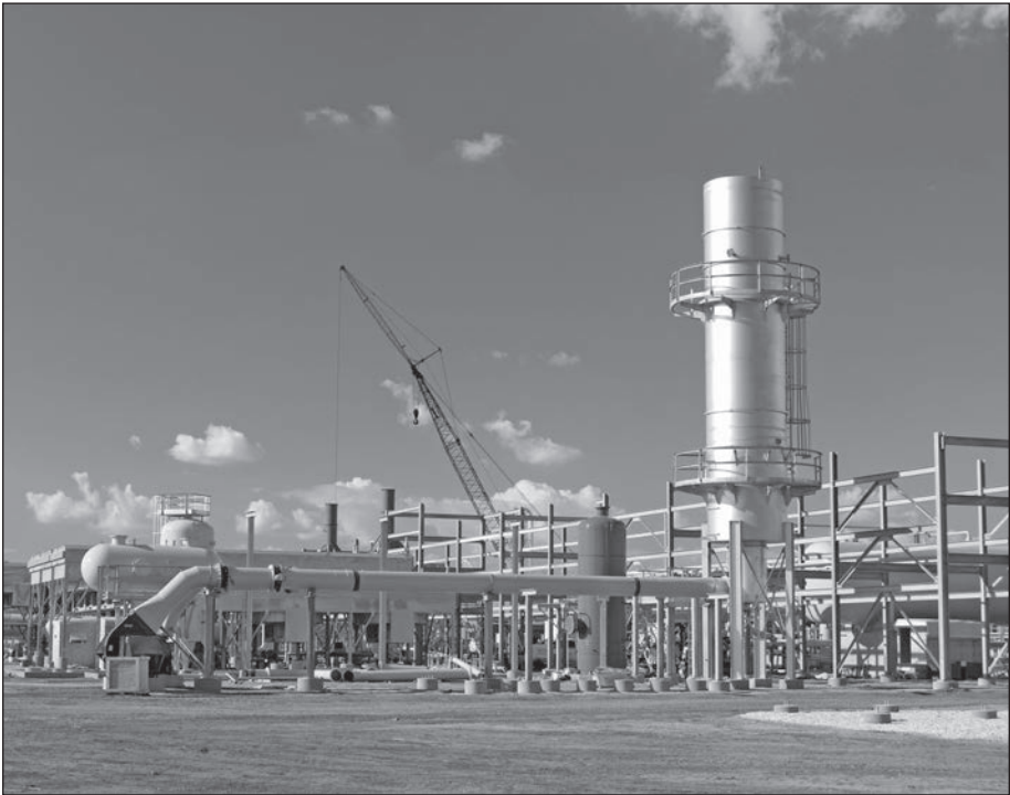
Fig. 11–2. Enterprise Products' gas plant at Yoakum, Texas. Processing nearly a billion cubic feet per day, the plant produces about 111,000 barrels per day of NGLs.
