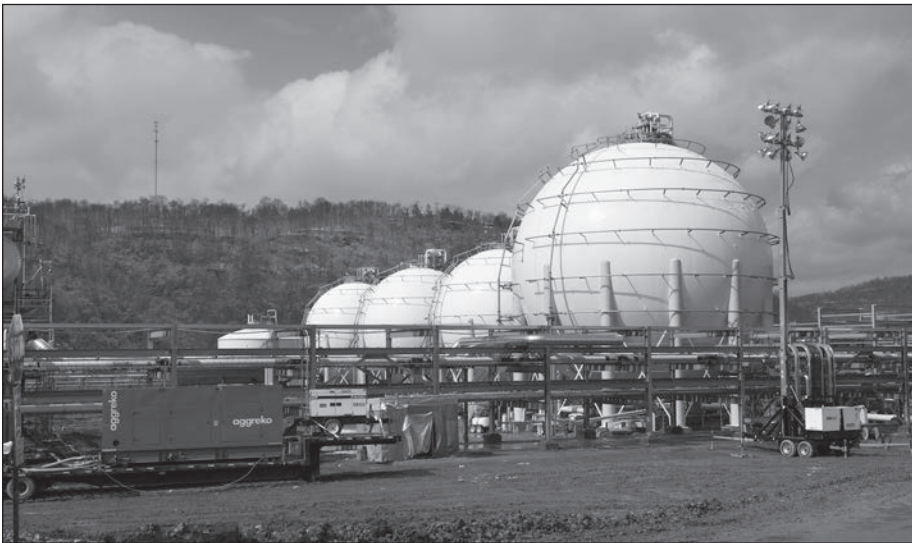
Fig. 7–9. Steel spheres for propane storage (courtesy of Dominion)
