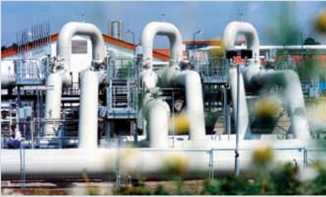
Wingas compressor station, Eischleben, Germany: Two Siemens compressor trains, each powered by a 30MW SGT-700 gas turbine, boosting the pipeline pressure for Natural gas* transport.
