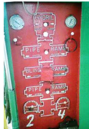
شکل 10 : BLOWOUT PREVENTER CONTROL UNIT
