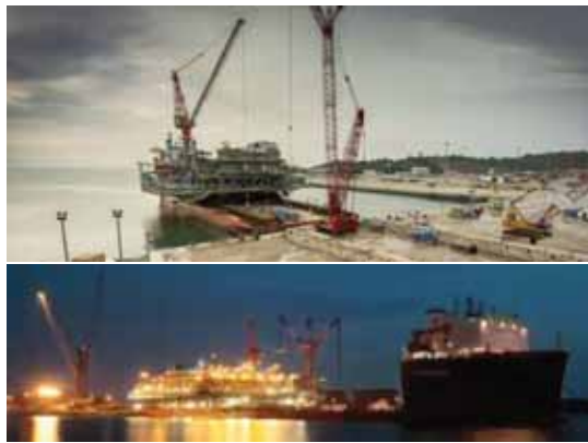
Central Metering and Manifold Platform Loadout – Iraq Crude Oil Export Expansion Project, South Oil Company
