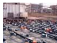
Electrochemical Remediation Technology
