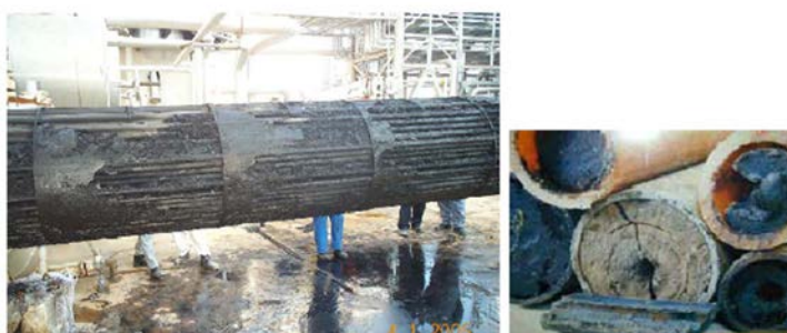
Heat exchanger bundle and pipelines plugged with asphaltenes
