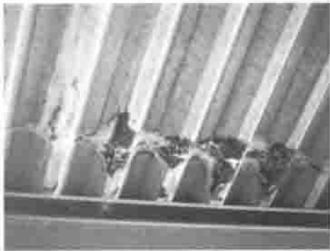
Fig. 1 Corroded steel formwork on the ceiling of a parking garage. The seams in this corrugated structure act as condensation traps and lead to wet atmospheric corrosion. Courtesy of R.H. Heidersbach, California Polytechnic State University
