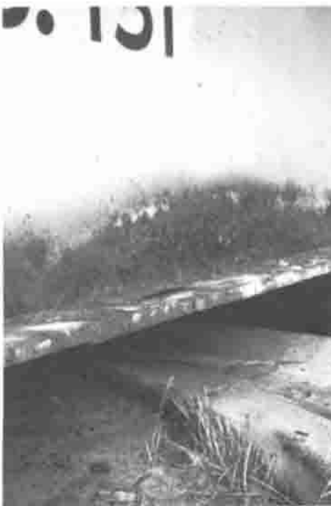
Fig. 4 Corroded weathering steel highway bridge girder. Courtesy of D. Manning, Ontario Ministry of Highways and Communications
