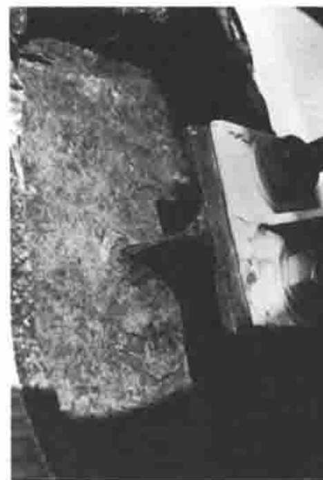
Fig. 7 Heavy corrosion of a steel support bracket where it passed through cellular glass insulation on a cold-temperature column. Moisture condensed on the column shell where the support was warmed by the extended attachment.
