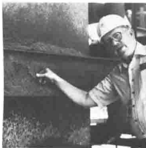
Fig. 6 Delamination of plain carbon steel due to \text{SO}_2 + ash deposit outside the boiler area of a coal-fired power plant. Courtesy of D.M. Berger, Gilbert/Commonwealth
