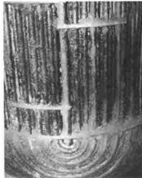
Fig. 5 Fouled heat-exchanger tube bundle
