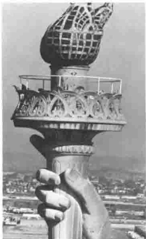
Fig. 10 Rust staining of the Statue of Liberty torch due to galvanic corrosion of the iron armature in contact with the copper skin. Courtesy of R. Baboian, Texas Instruments, Inc.
