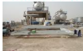
Accumulator and Flash drum PSV platform assembly
