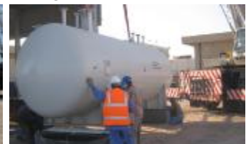
DS1 Instrument Air Receiver installation
