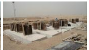
Metering Skid Foundation Pedestal
