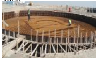
Crude Oil buffer tank foundation
