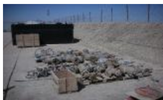
Failed equipment changed on existing wells to restore integrity
