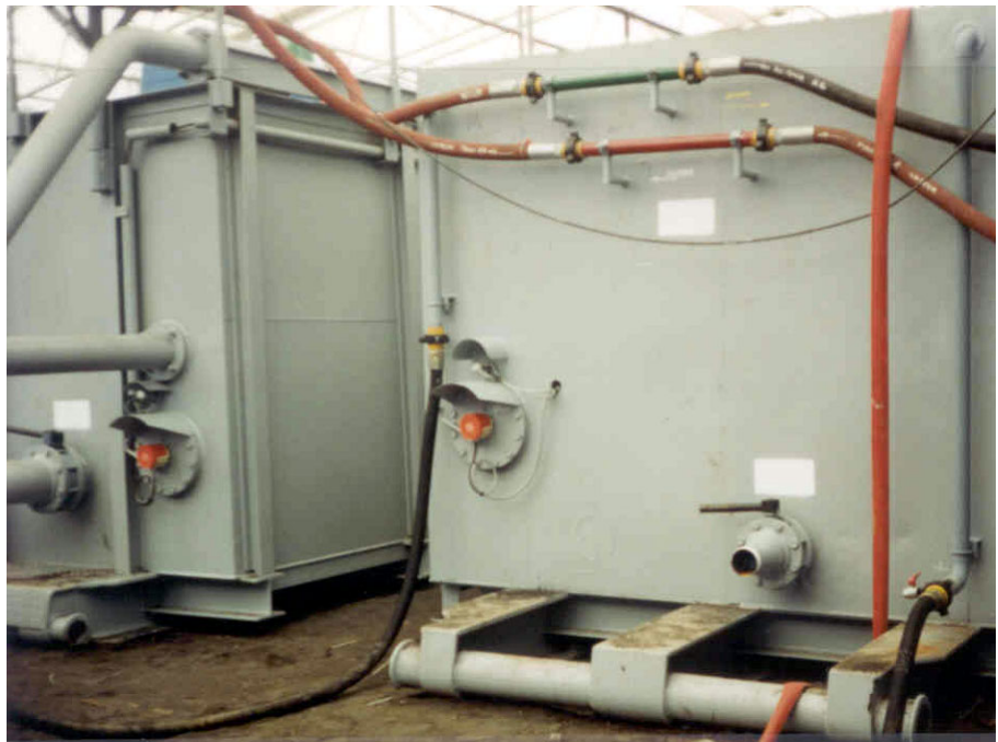
Electric resistance heating
