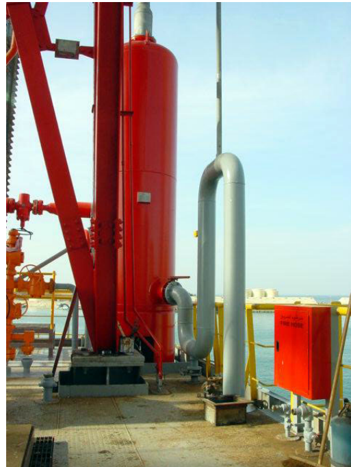
Mud gas separator
