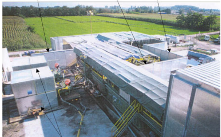
Complete covering on mud pumps' engines
