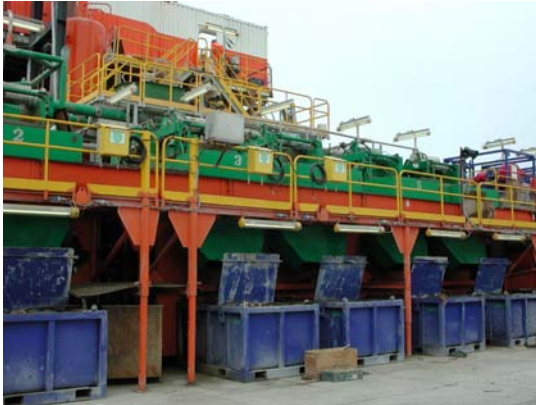
Solids Removal Systems
