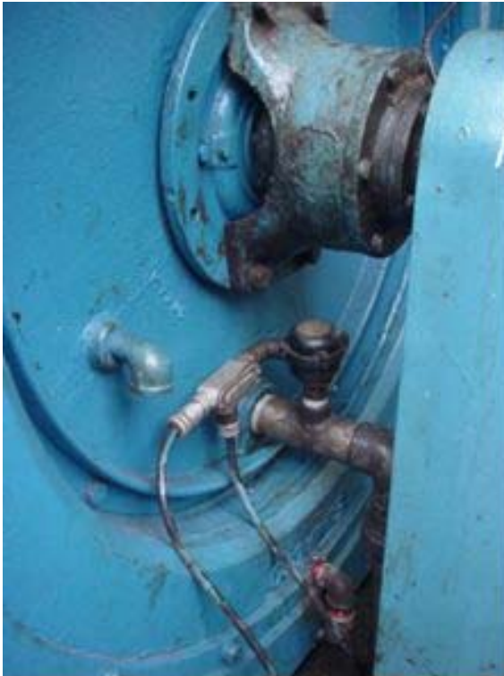
Figure 6 - Flow and temperature sensors.
