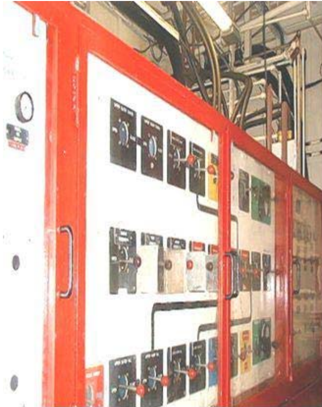
Figure 13 - BOP HPU Cameron-Payne control systems.
