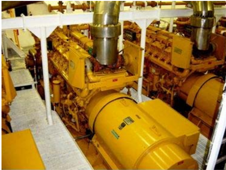
Figure 2 - Example of a clean and tidy engine space.
