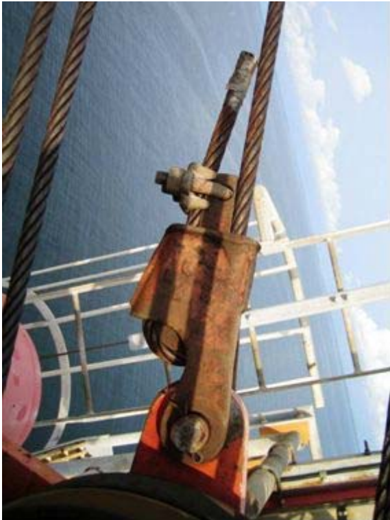
Figure 25 - Well secured Wedgelock.
