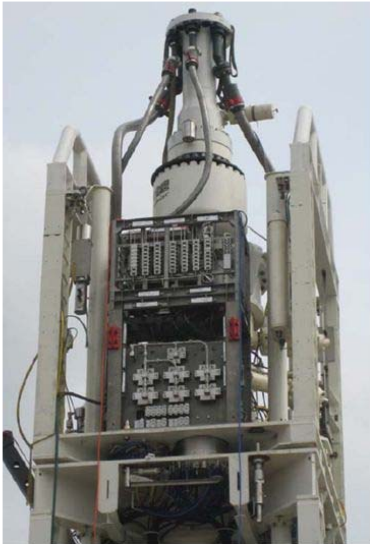
Figure 15 - Cameron MUX Mk III control pod.
