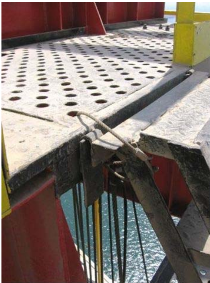
Figure 38 – Platform with safety wire across the hinge.
