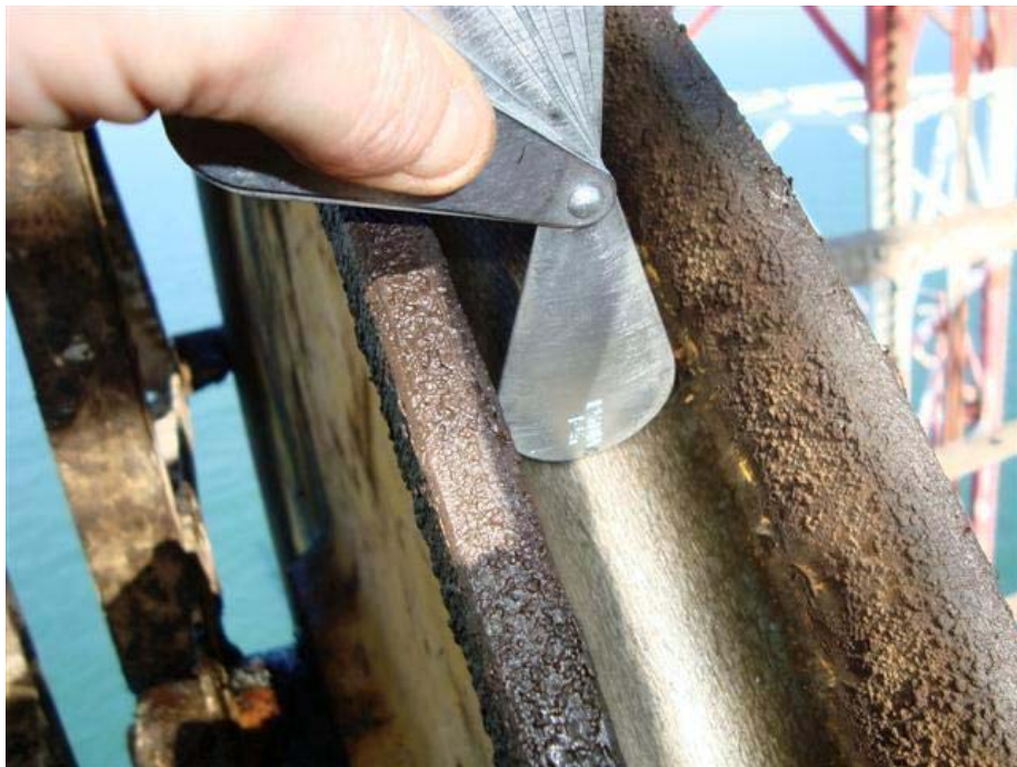
Figure 25 - Measuring the sheave wear.
