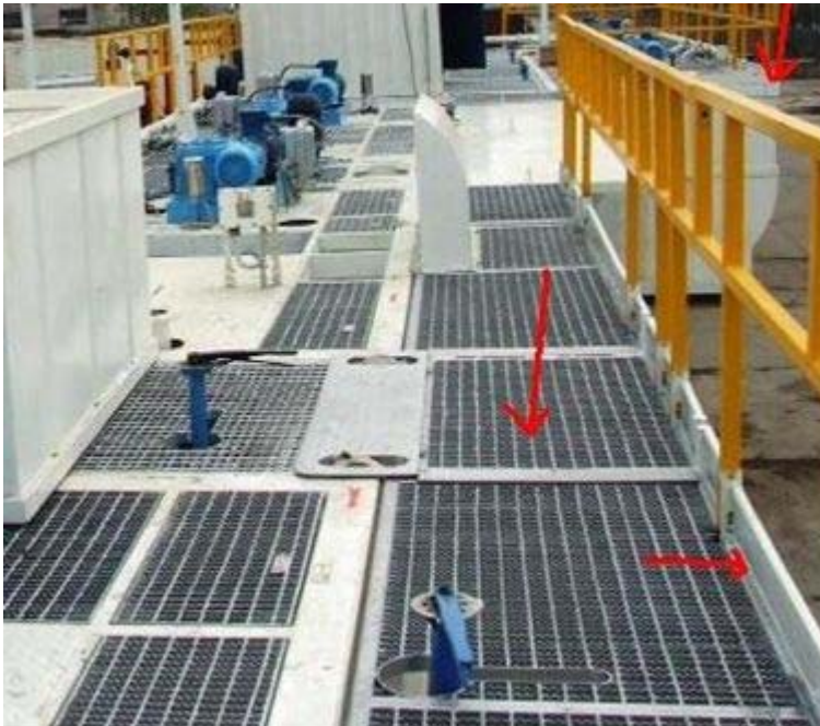
Figure 7 - Mud pit with secure grating and proper toe boards.
