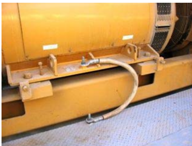
Figure 9 - Substantial ground cable for generator.
