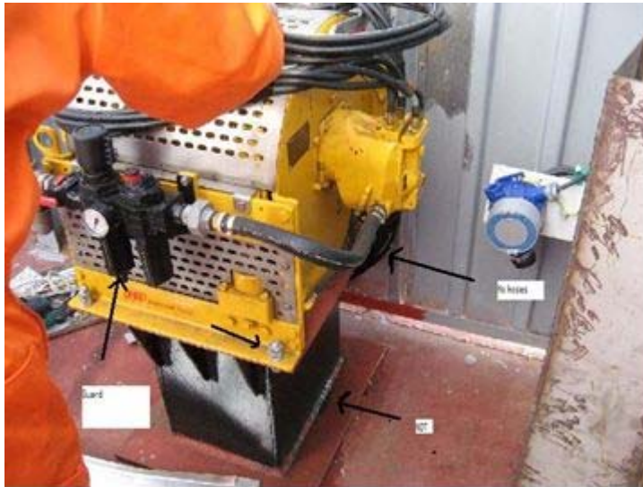
Figure 44 - Poorly fitted man-riding winch.
