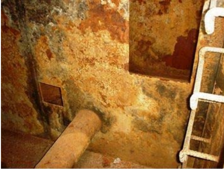
Figure 28 - Badly corroded mud pit walls.
