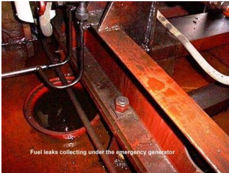
Figure 9 - Fuel leaks under the generator constitute a fire hazard.
