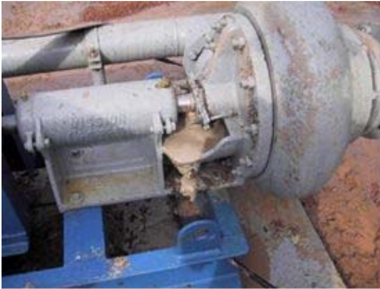
Figure 20 - Centrifugal pump: gland packing.
