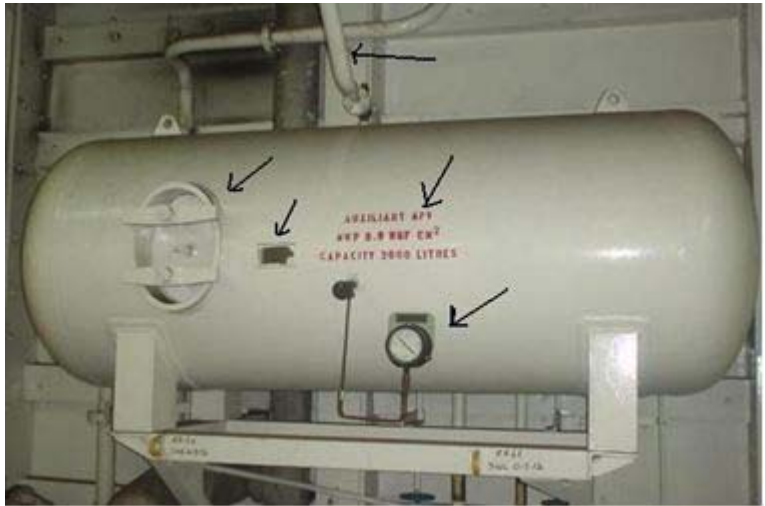
Figure 16 - Typical air receiver.
