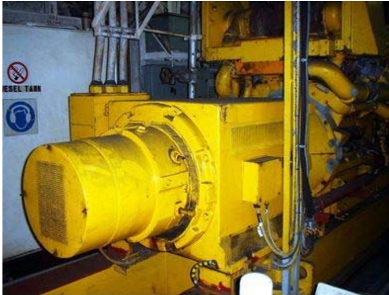
Figure 7 - Emergency generator engine
