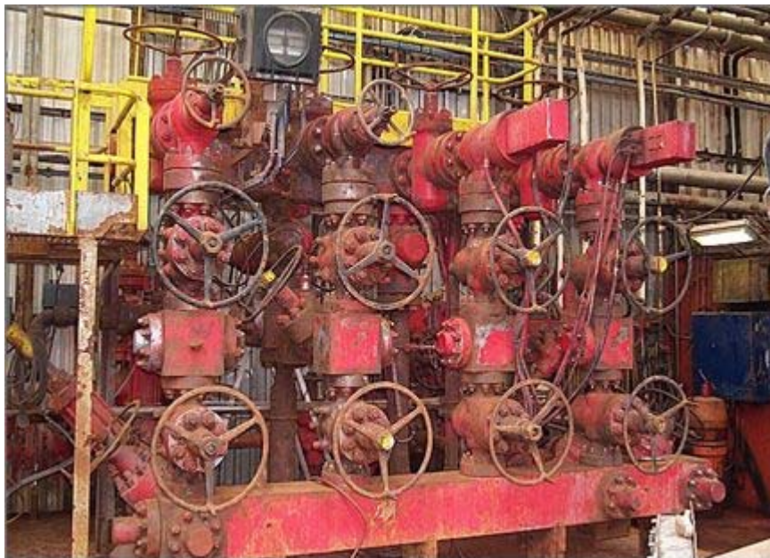
Figure 10 - Choke manifold with a single high-pressure buffer tank, which is not API-recommended.
