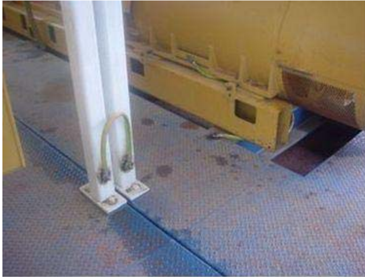
Figure 7 - Electrical ground system.
