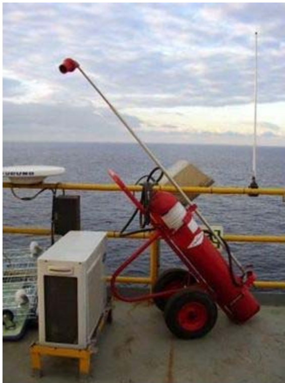
Figure 3 - Fire extinguisher with extension nozzle.
