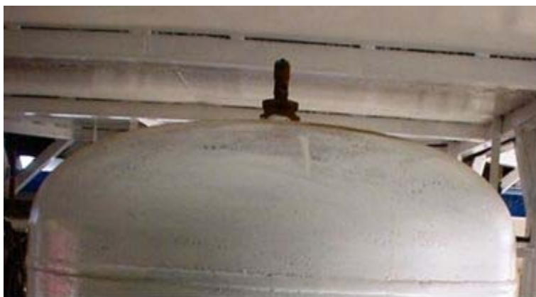
Figure 15 - The size of the relief valve is important.
