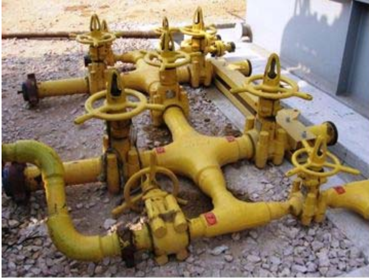
Figure 18 - Numbered ground manifold.
