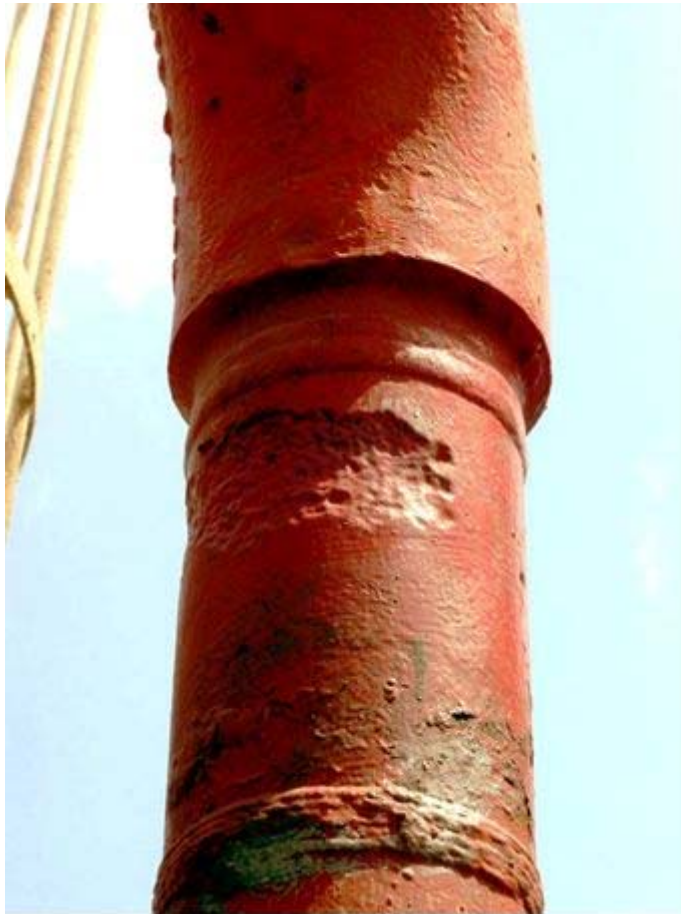
Figure 16 - Corrosion is not just an internal problem.
