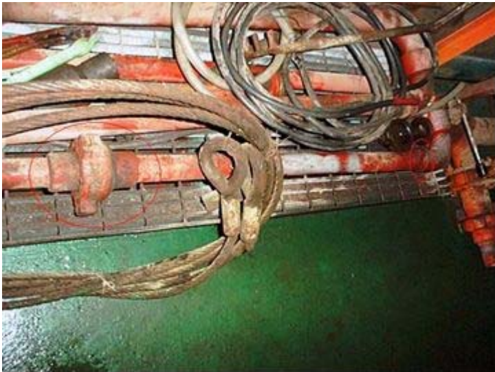
Figure 19 - Chiksan union without safety sling.
