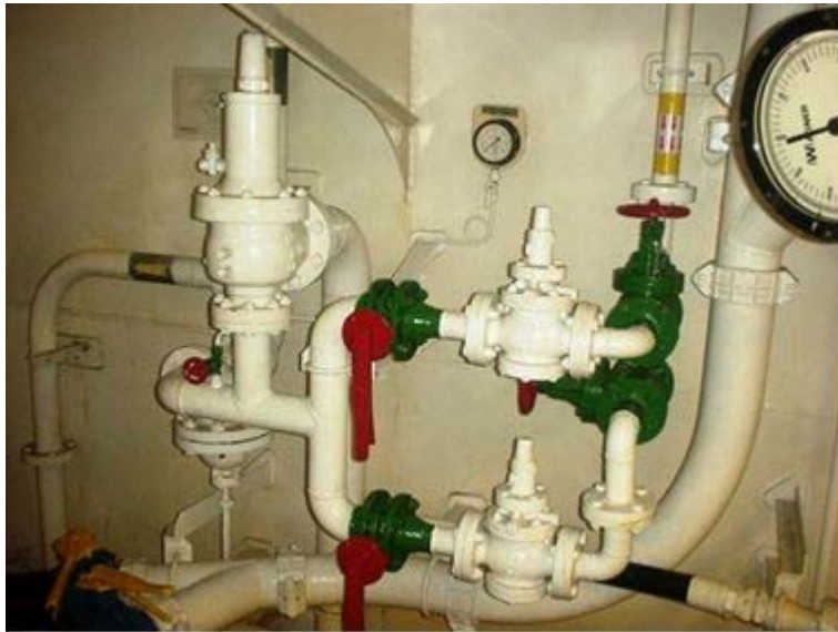
Figure 13 - Bulk air reducing station.
