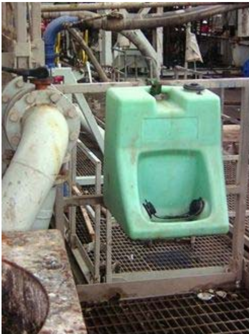
Figure 29 - Typical eyewash station.
