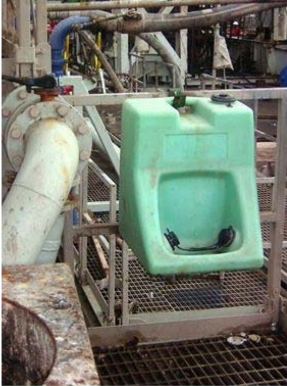
Figure 6 - Typical eyewash station.
