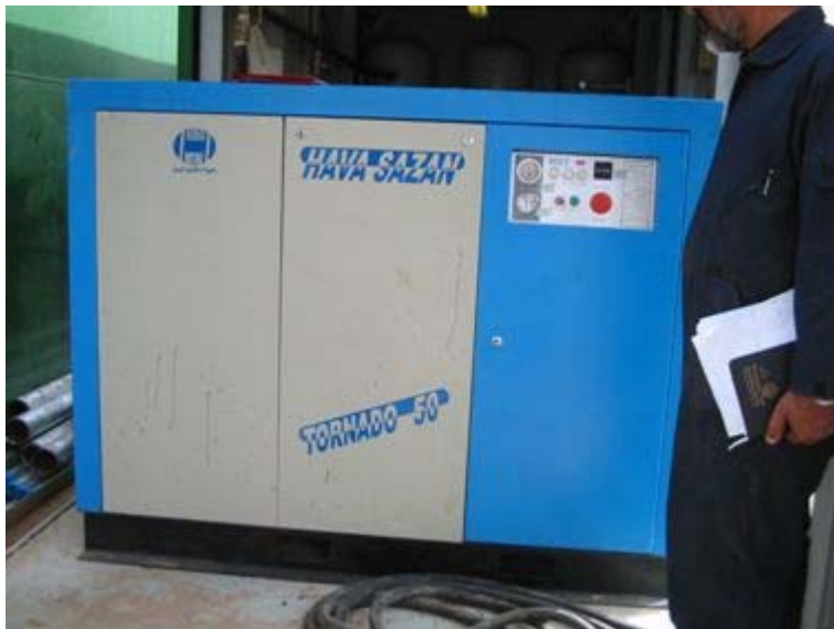
Figure 14 - Typical modern air compressor.
