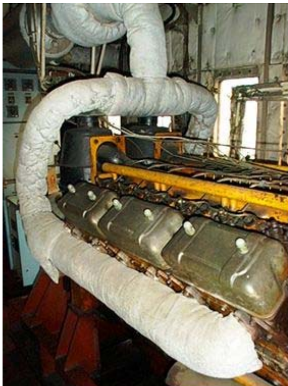
Figure 3 - Example of good exhaust insulation.
