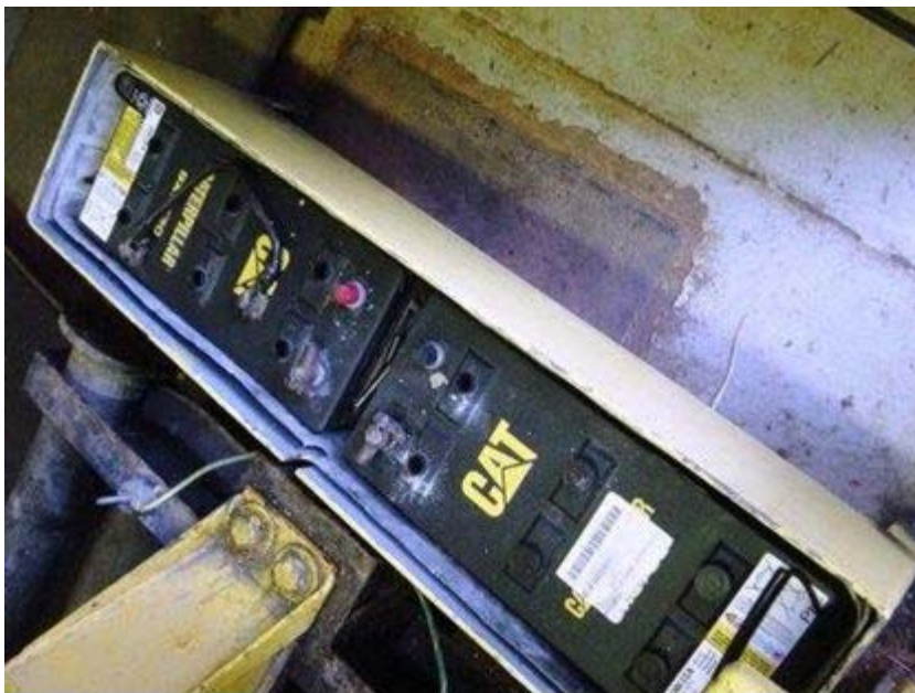
Figure 11 - Neglected starting batteries; these must be kept in good condition.
