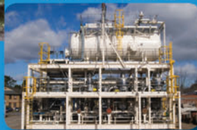
Produced Water Treatment
