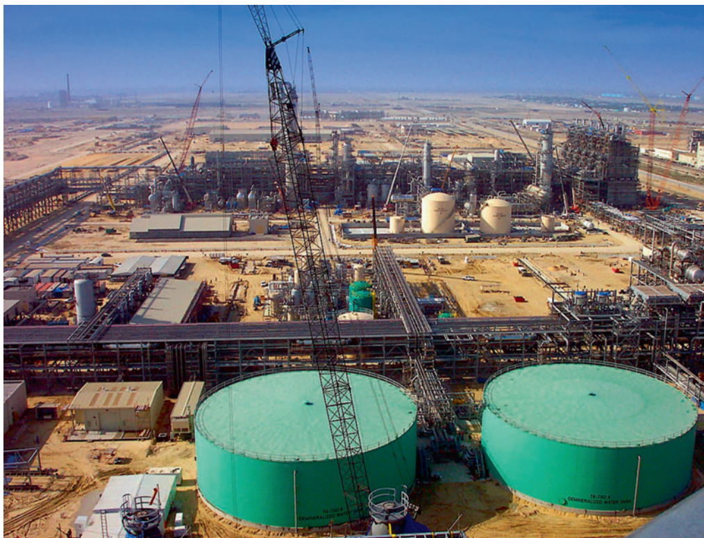
Fluor's goal is to provide integrated, capital-efficient projects locally while maximising supply chain efficiencies. (Photo: Fluor)
